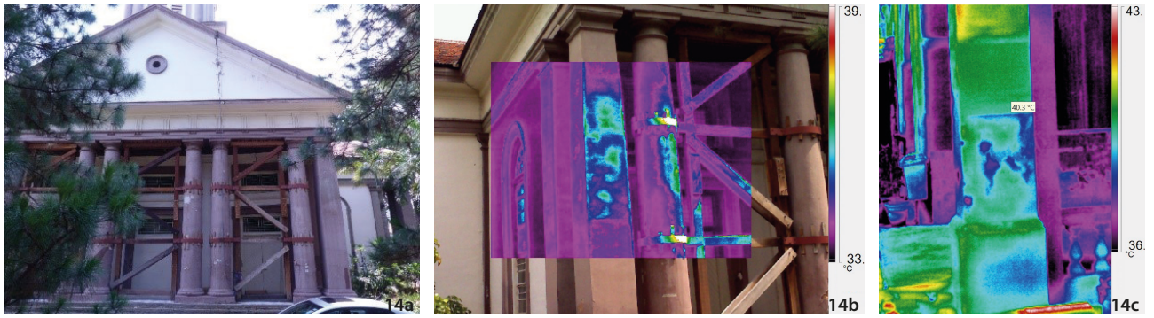
Figure 14 The left photo shows a section of the Cathedral of Good Shepherd. The centre and right photo show thermograms captured with thermal anomalies. The irregular cold spots are an indication of deteriorated and debonded render. A regular hotter area above the irregular cold spots in the right photo is due to the presence of latter applied cement-based render. This was applied apparently to address the deterioration of the historic render caused by the salt attack (Source: the author).
