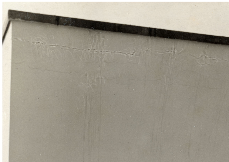
Fig. 7 Tugendhat House, Brno 1930, south east wall of Grete Tugendhat's dormitory, detail: the crack between concrete roof and the brick wall, a deficiency in the construction, has been retouched (Source: Rudolf de Sandalo, Brno 1931, detail)
