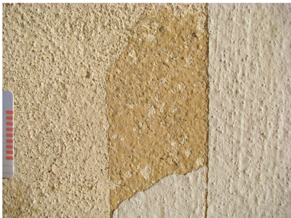
Fig. 9 Tugendhat House, Brno, 1930, view to the southeast, detail: probe during the removal of the later plasterings (from right to left): painting of 1985 (with cement and synthetic resin), two lime coats (between 1945 and 1965), heavily sulfated due to air pollution, and original surface with yellowish whitewash (picture lower edge approx. 17 cm) (Source: Ivo Hammer 2011)
