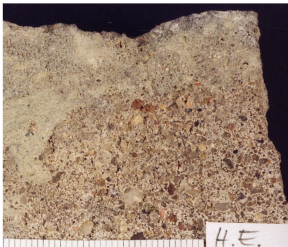
Fig. 11 Ludwig Mies van der Rohe, Berlin Nicolasse, Dreilindenstraße 30, Haus Eichstaedt (1921–1923), plaster sample: rubbed reddish-yellow plaster (with brick fragments and partially preserved patina) (Source: study work HAWK / Hildesheim, Ivo Hammer, Stefanie Dannenfeldt, Vanessa Knappe, Natalie Schaack)
