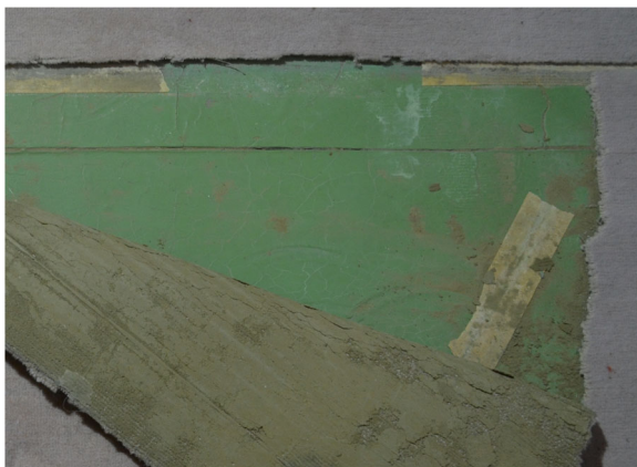
Fig. 26 Josef Frank and Oskar Wlach, House Beer in Vienna Hietzing (1930), attic, northern room with largely preserved green rubber flooring (Source: Ivo Hammer 2017)
