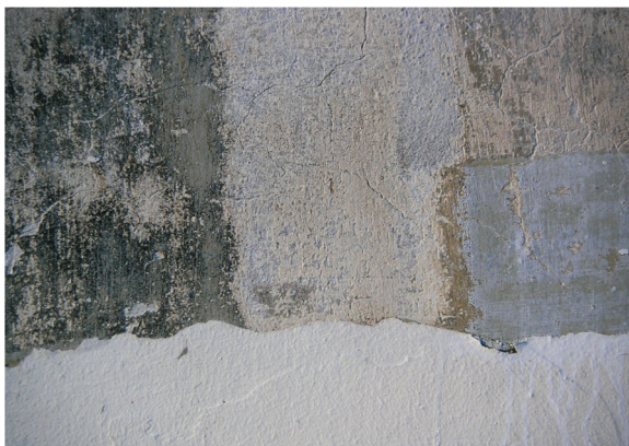
Fig. 13 Walter Gropius, Dessau, Bauhaus, Prellerhaus, 1926, east facade, detail, samples for the removal of later coatings; on the smoothed reddish-yellowish plaster (early shrinkage cracks!) lies a thin lime wash of the same colour, probably dyed with silicate sand fines. The surface is patinated and also sulfated (Source: Analysis Nils Mainusch, HAWK / Hildesheim, 2000)
