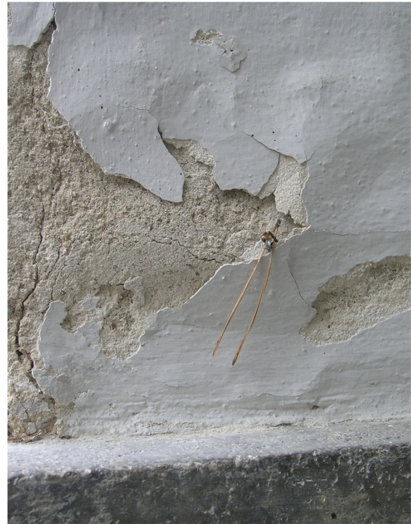
Fig. 14 Dessau, master house Klee / Kandinsky, 1926; the original material-coloured smoothed plaster appears under the recent titanium-white coating, possibly containing a synthetic resin component, in 2006 (Source: Ivo Hammer)
