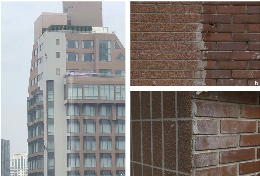
Fig. 14 Exterior facade coated with lacquer (construction site and details) (Sources: a Fan 2018; b, c Wu 2018)
