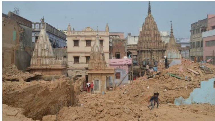
Fig. 3 Demolition work for the Kashi Viswanath Temple Corridor, Varanasi (Source: Tarique Anwar)
