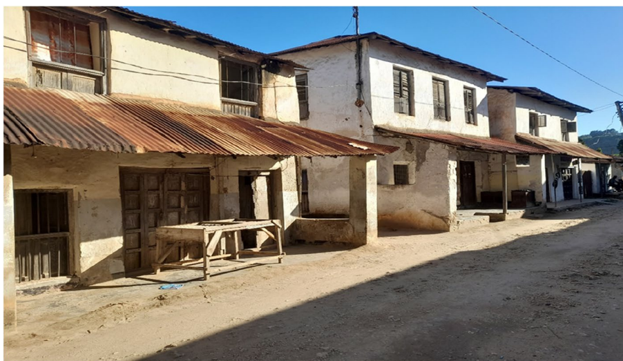
Fig. 5 Some built heritage sites along Indian Street in Pangani Historic Town (Source: the authors)
