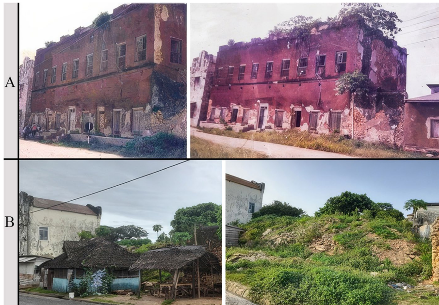
Fig. 6 Al Kassaby building, previously used as a CCM office in Pangani, now in ruins (Source: the authors)
