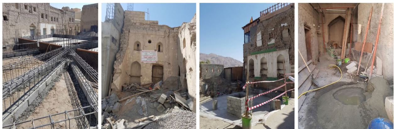
Fig. 10 Location and photos of the ongoing constructions in Harat al'Aqr (March 2021) (Source: Google satellite image, enhanced by the author)
